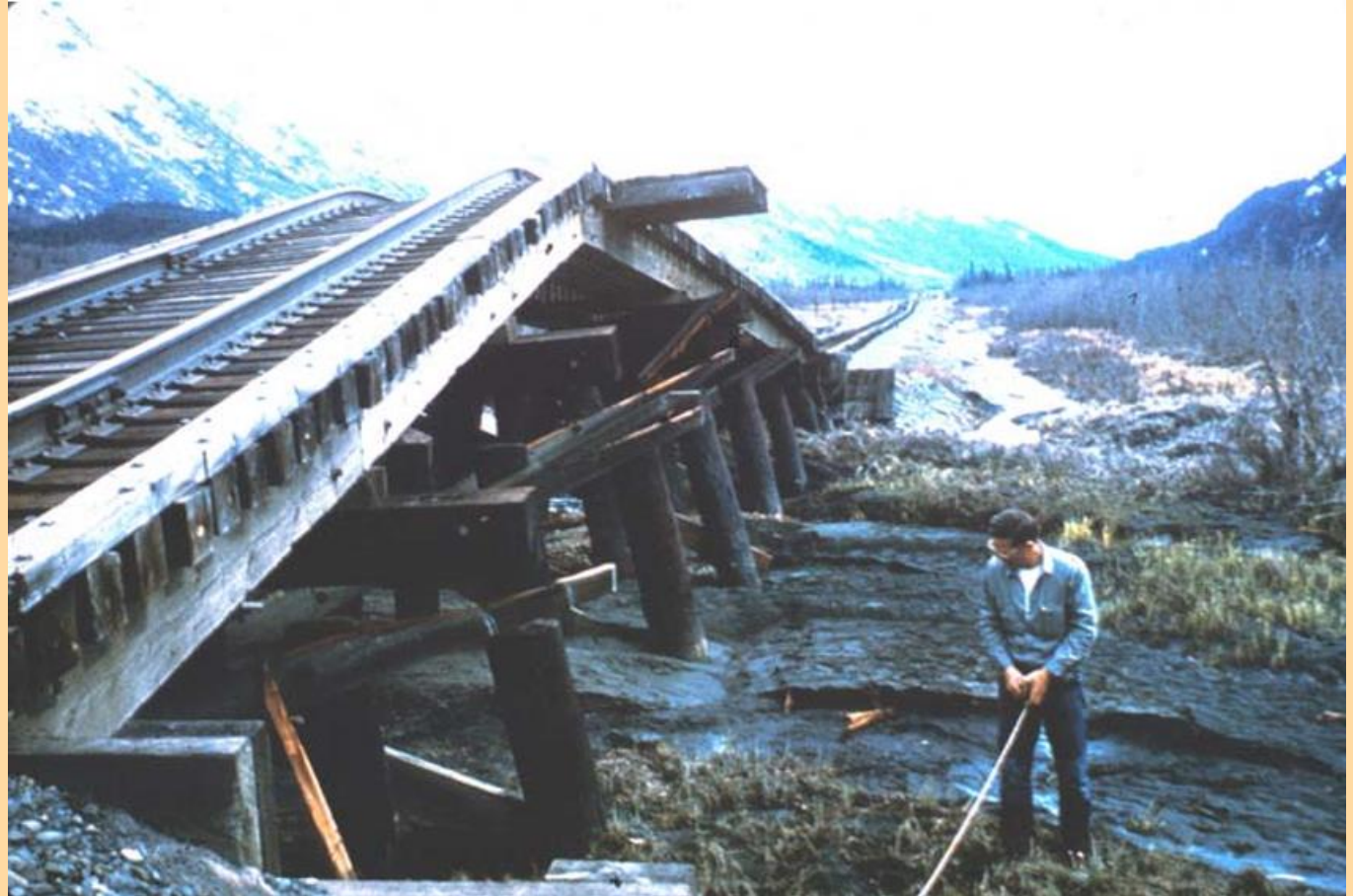
Iron road on Kenai River after Alaska Earthquake, 1964
