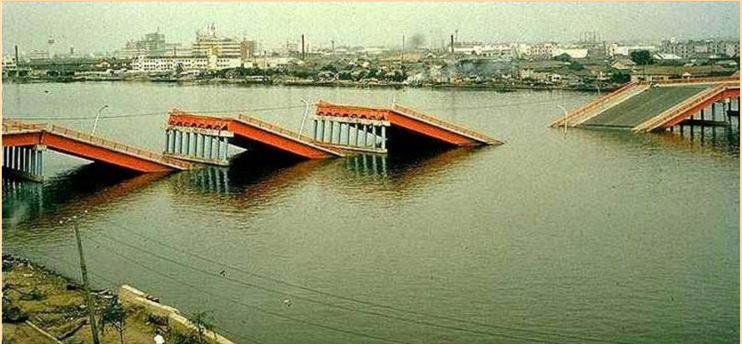
“Showa” Bridge after Niigata Earthquake, 1964, Japan
