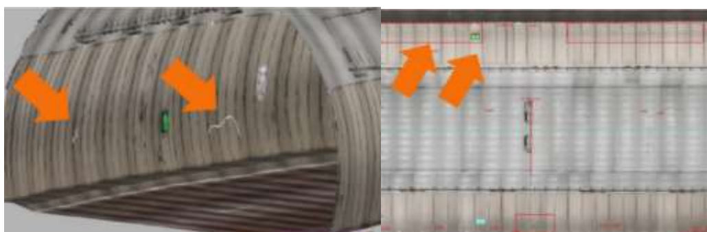
Figure 2.14 An example from a photo of tunnel lining projected on to a BIM model (left) and a orthogonal photo with detected cracks (right); ASFINAG, Austria.
