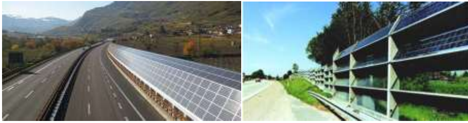
Figure 6.12 Examples of barriers with photovoltaic panels installed in Brennero Italy; [58].
