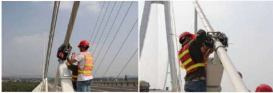
Figure 4.10 Inspection of Nanjing 3rd Yangtze River Bridge with Cable-climbing robots; JSTI Group China.
