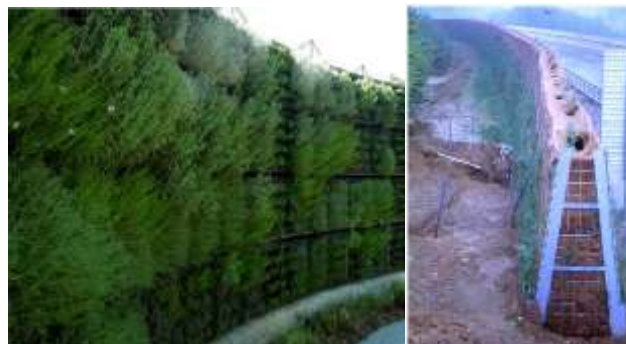
Figure 6.11 Examples of barrier types: Green Wall (left) and Bio-barrier in construction (right).
