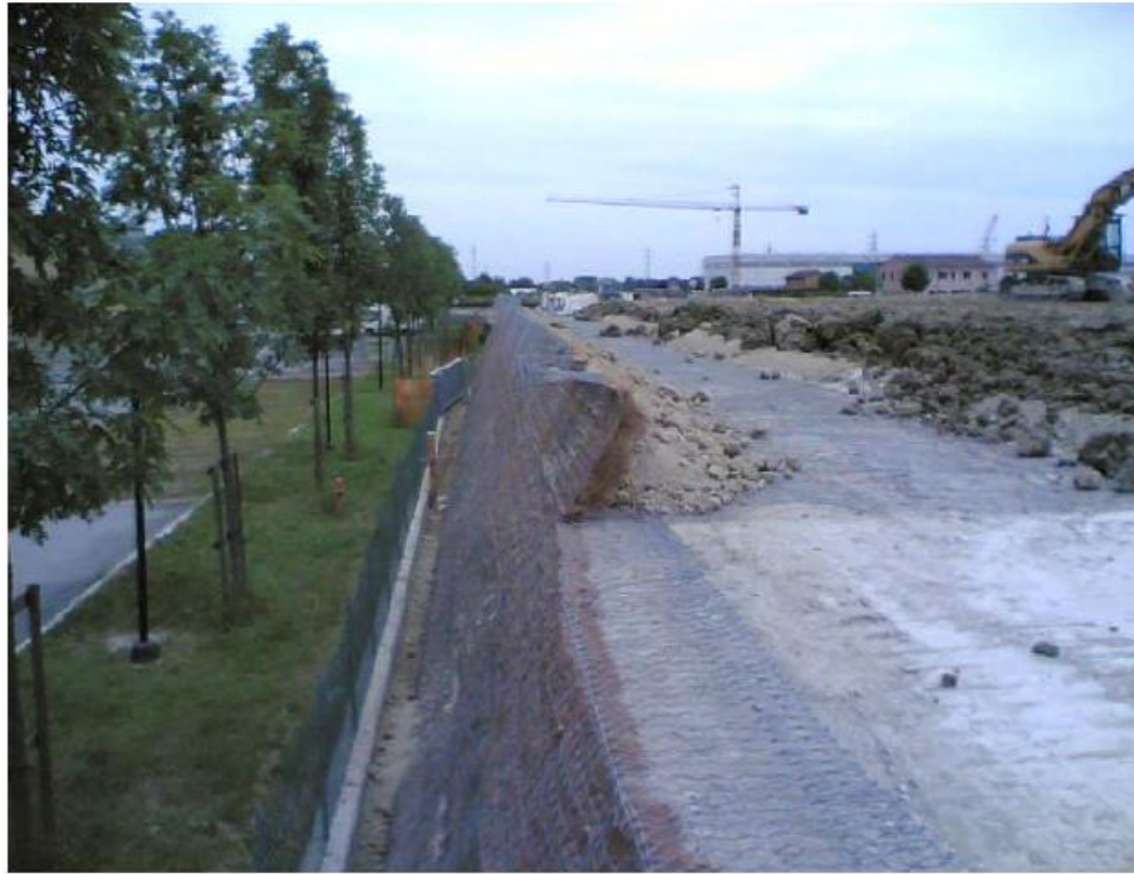
Figure 7.2: . Tangential Road of Forlì (Italy) – Embankments with lime-treated materials and Reinforced Earth Walls.
