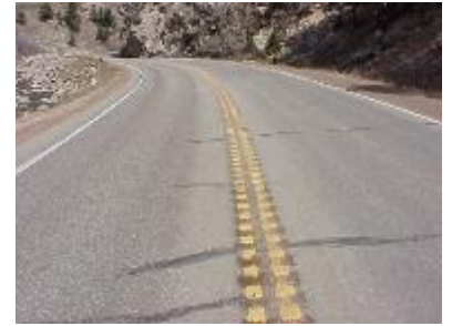
Figure 2.16 Centerline rumble-stripe in USA, Source: FHWA
