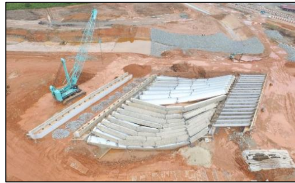
Figure 7 (b) : Aerial view of the total collapse of the beam
