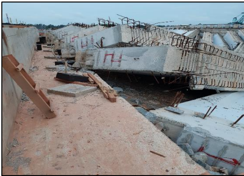
Figures 7 (a): Precast beam collapse in domino effect due to the stability issue
