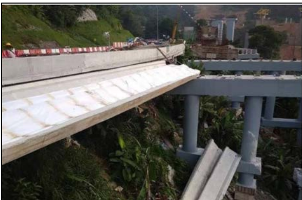
Figure 7 (c) : Precast beam collapse at construction site
